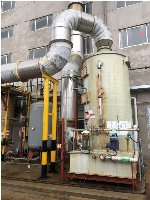
B40 车间（一楼）室内换风-一级水喷淋
