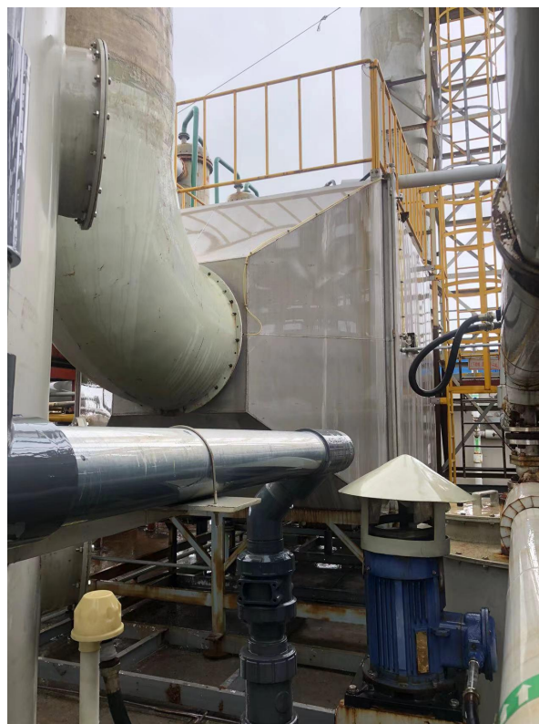
B40 车间（顶楼）室内换风-一级活性炭吸附
