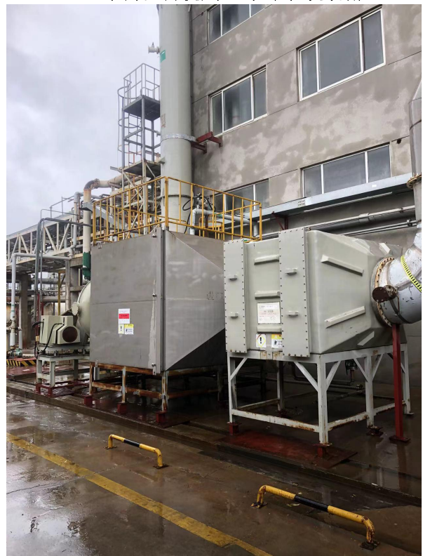
B40 车间（一楼）室内换风-一级活性炭吸附
